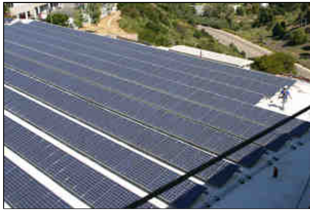
The building's solar arrays will provide nearly 20 percent of the building's electrical use.
